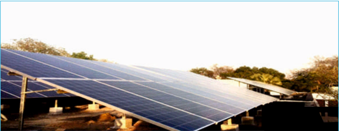
Solar Panel at Nursing Hostel
