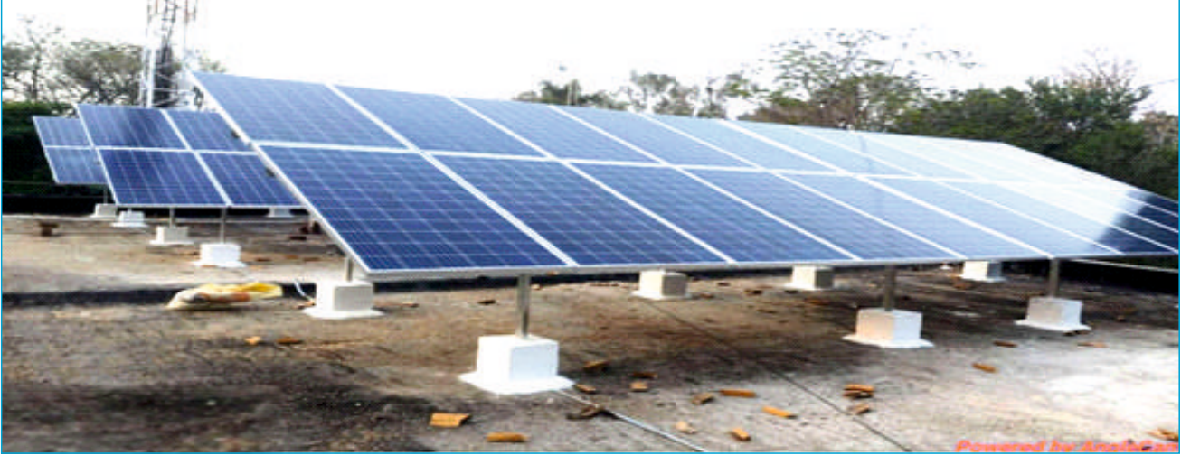
Solar panel at CCWO, office
