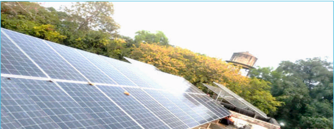
Solar Panel at Jagjivan Nagar Guest House
