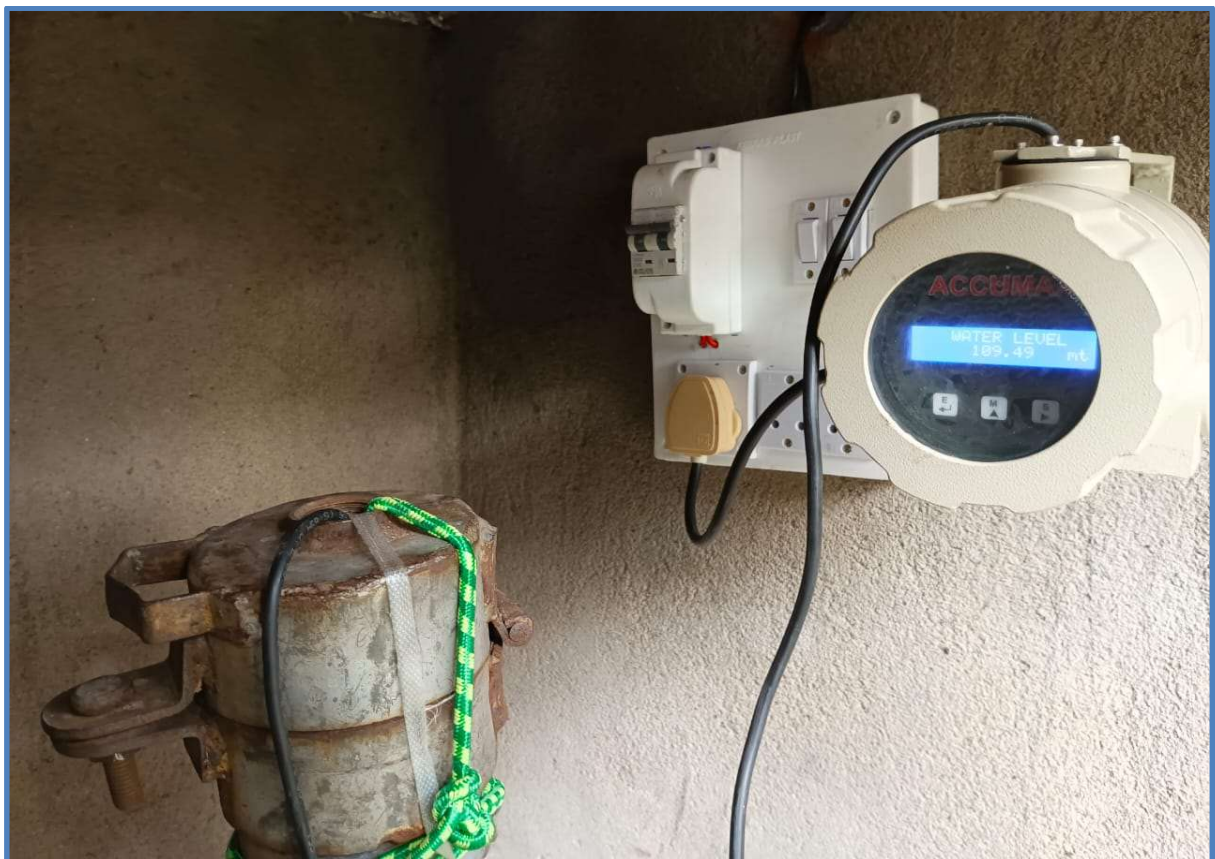
Picture 9 – Piezometric well with DWLR Cluster VI shares the same aquifer with cluster V and Cluster VII thus Pizeometers well of Cluster VII and Cluster V will be used for ground water monitoring.
