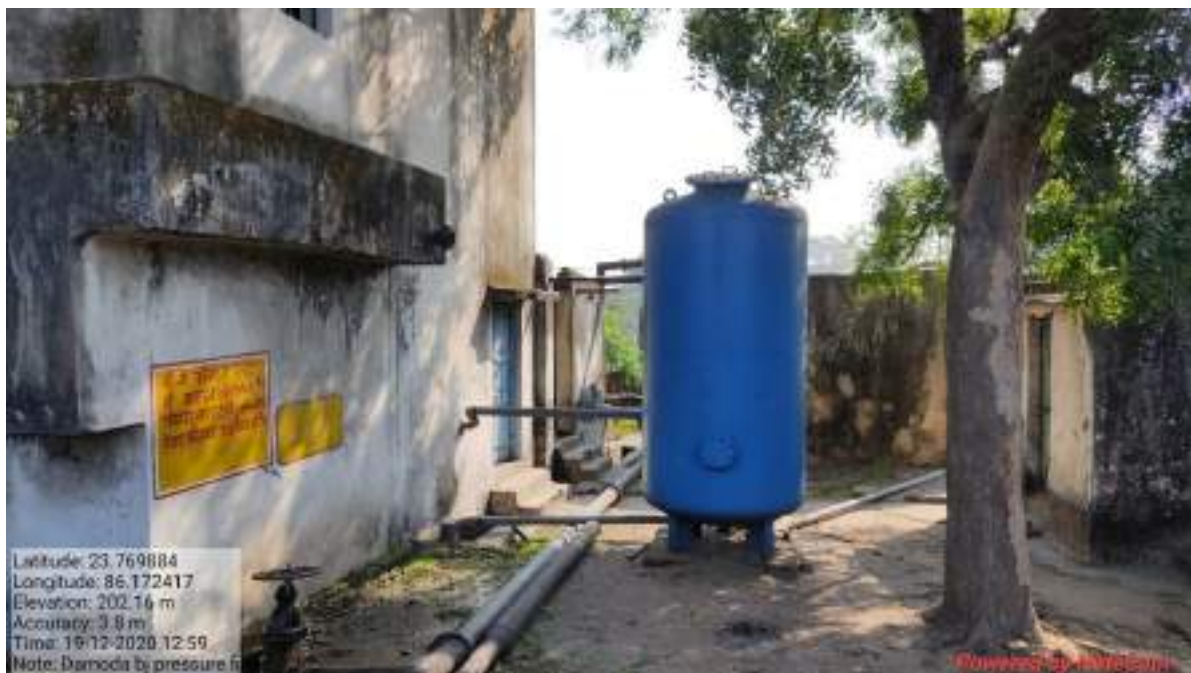
FILTER PLANT IN THE MINE AREA
