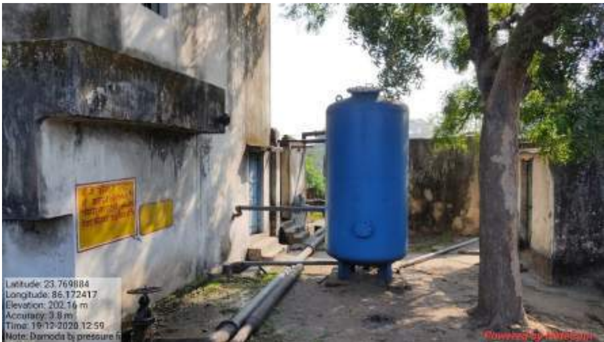
FILTER PLANT IN THE MINE AREA
