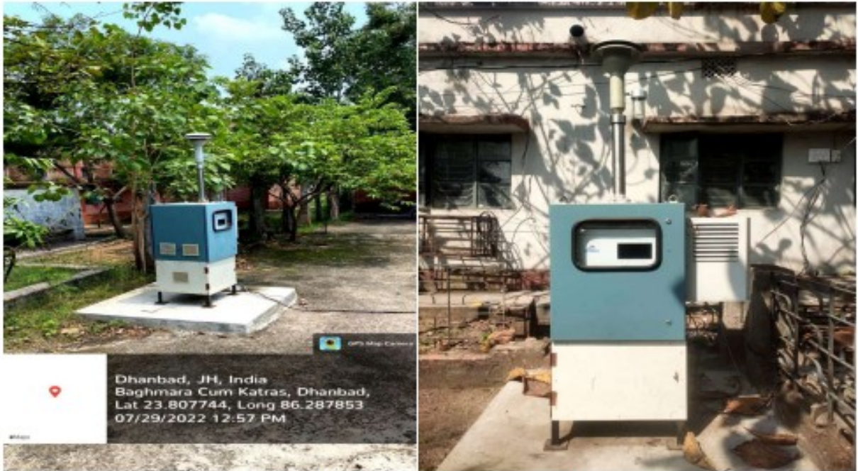
PM10 Online Analyzers installed at Collieries
