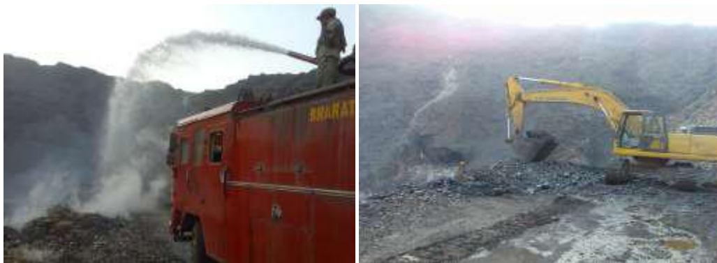
Fire excavation at Ena OC
